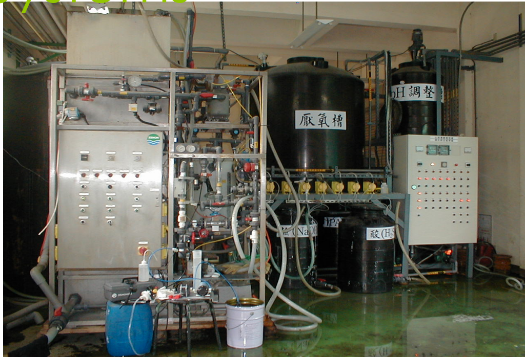
MBR Pilot System (Capacity: ~10m 3 /day)
