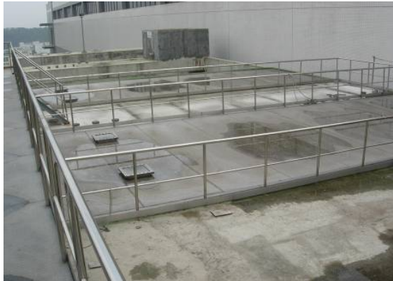
UASB Anaerobic System
