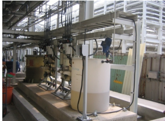
Chemical dosing station
