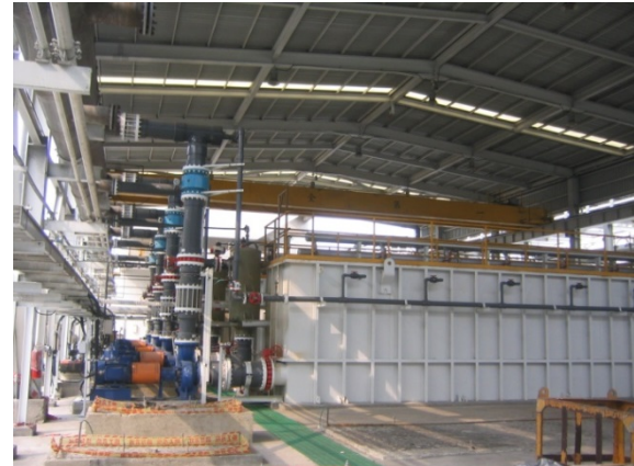
Membrane tanks and pumps
